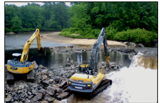
Removal of the Merrimack Village Dam in 2008. Photo courtesy Gomez and Sullivan Engineers, P.C.
